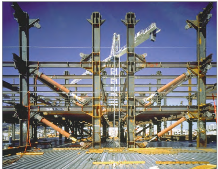
From kTalk by John Messner, Assoc. Professor, Penn State University Planning the implementation of BIM Through the Project Lifecycle
